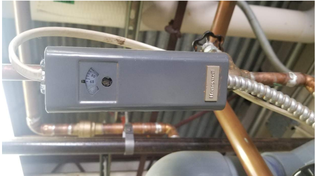
Aquastat for Domestic Hot Water Return
