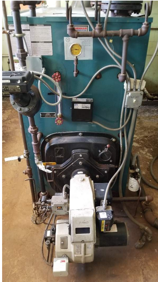
Existing Burnham boiler
