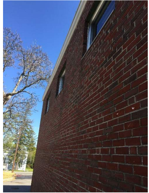
Exterior: windows out of plumb
