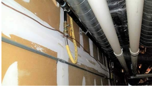
Gas Piping in Attic
