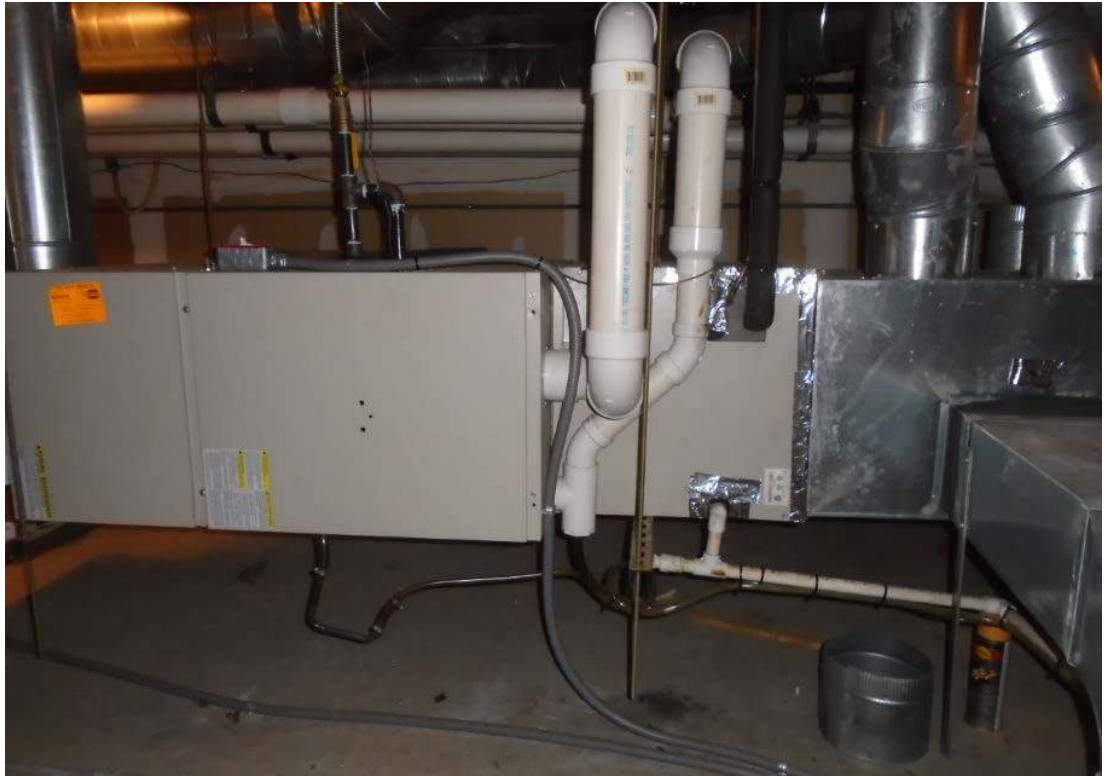
Existing gas furnace air handler and air conditioning coil
