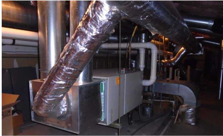
Example of Lossnay fresh air supply to return side of air handler
