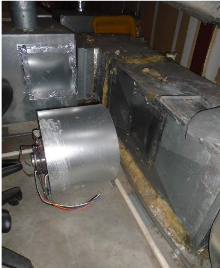
Example of uninsulated ductwork after modifications
