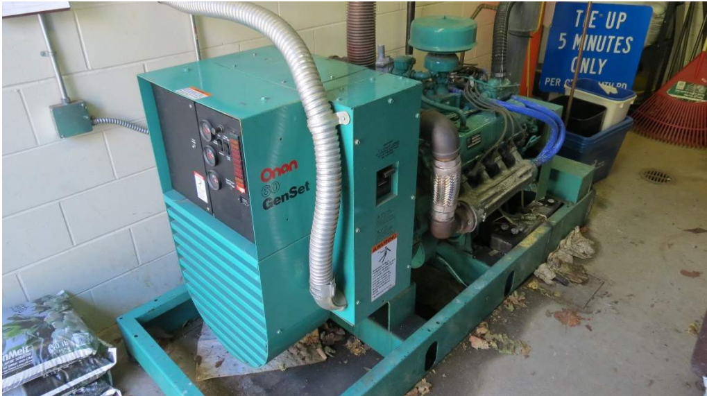
60kw diesel generator – Onan
