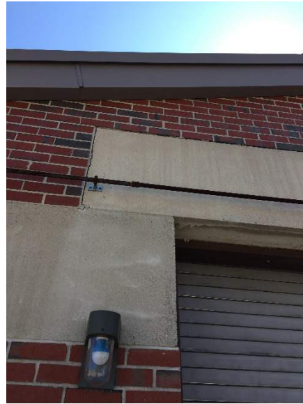
Cracking at precast concrete
