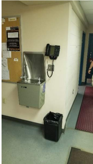
First Floor Water Cooler
