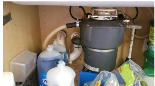
Disposal below Sink
