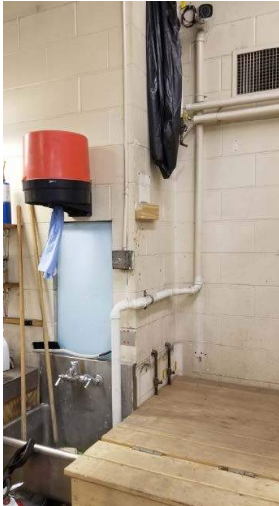
Condensate drain from attic to sink in cruiser garage
