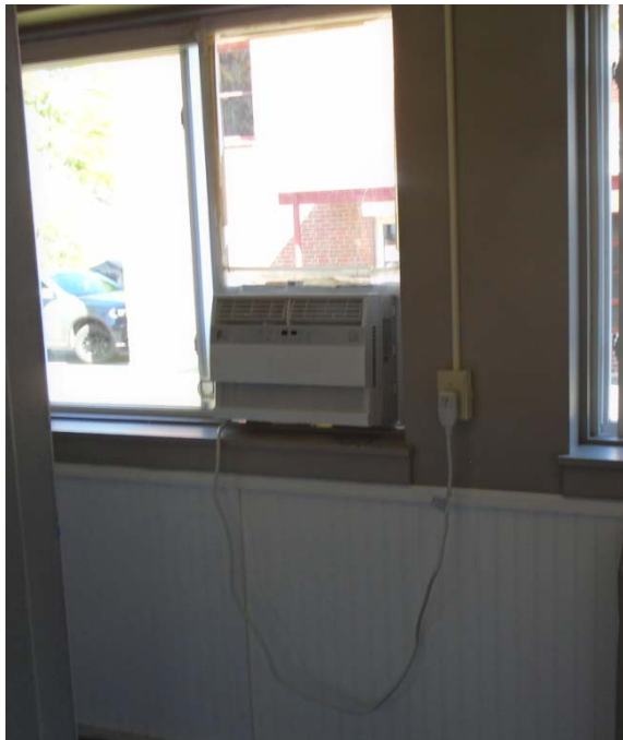
Window AC installed in the hallway outside of the bedrooms
