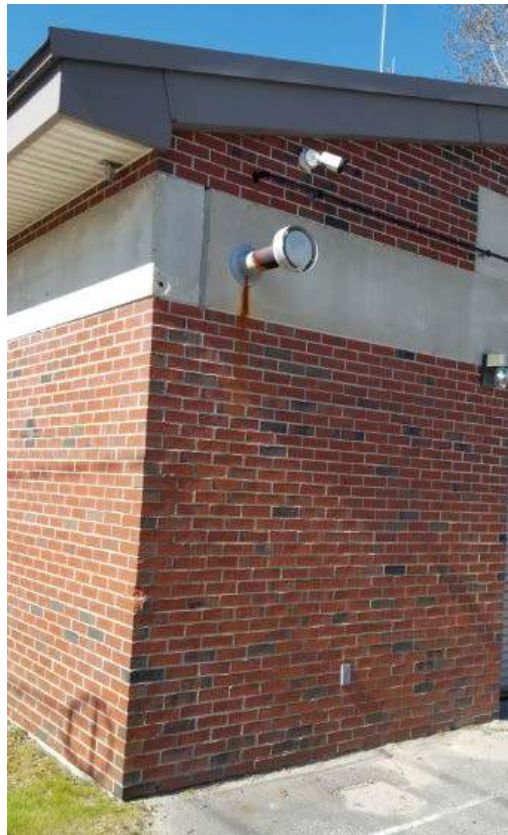
Exhaust vent on exterior of cruiser garage
