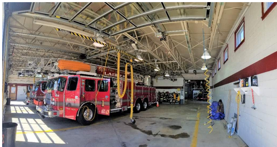
Main Three Garage Bays with Overhead compressed air and Water Fill Piping
