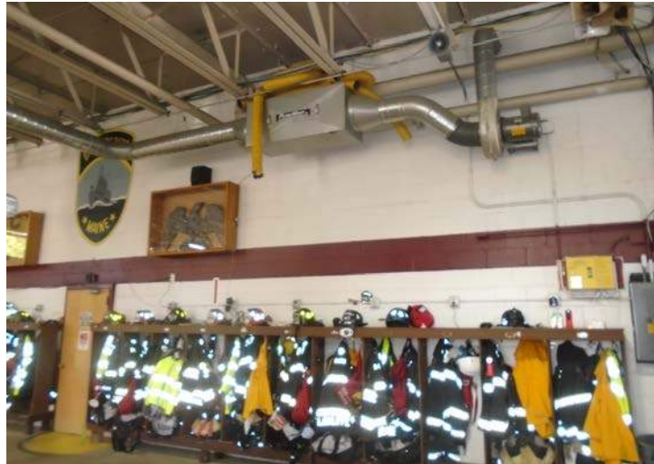
Plymovent system in main apparatus bay
