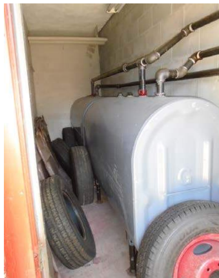
Oil Storage tank room
