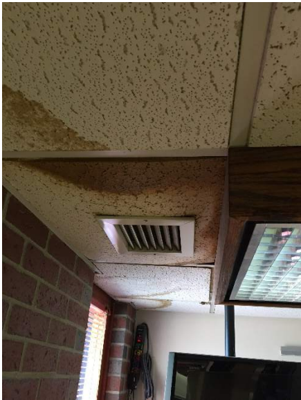
Interior water damage in conference room
