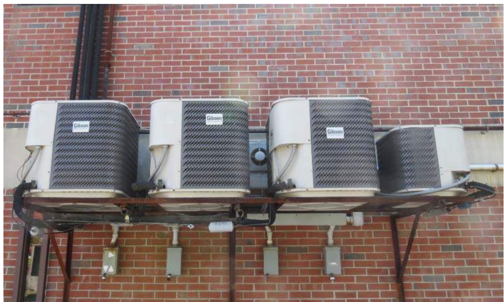
AC compressors installed on rear of building
