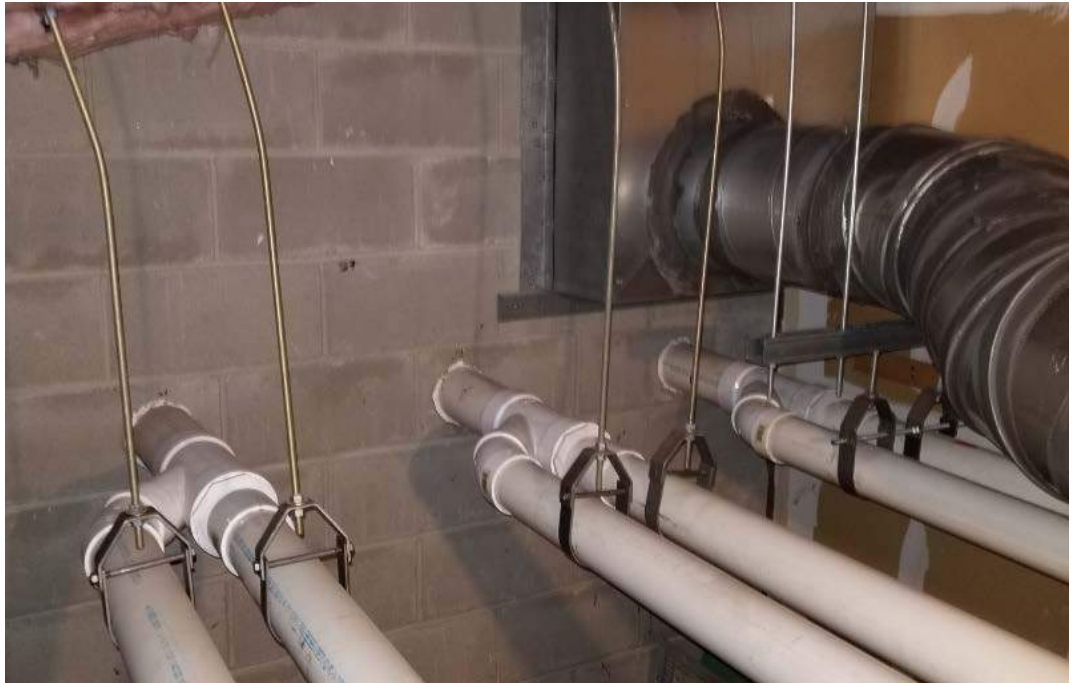
Exhaust and combustion air penetrations on side of building
