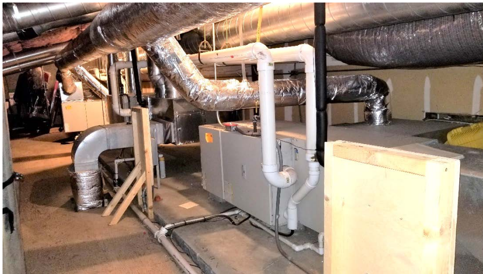
Attic Air Handling Equipment
