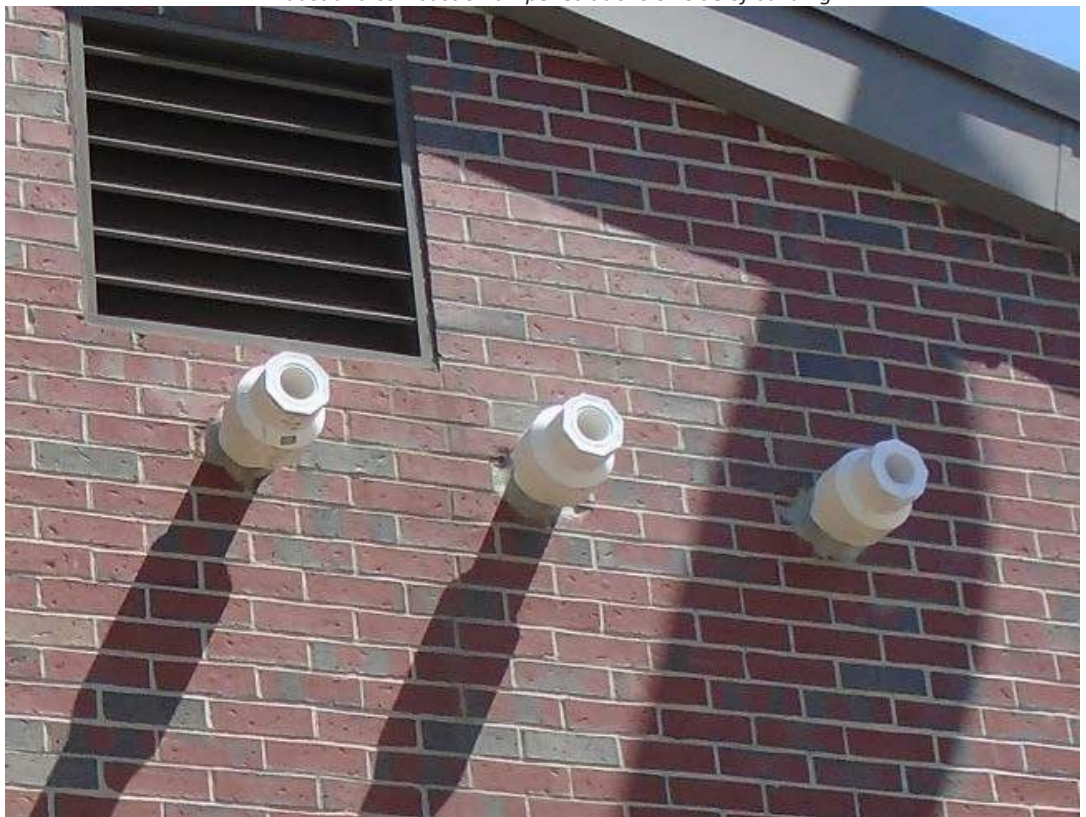
Coaxial exhaust and combustion air fittings on exterior of building
