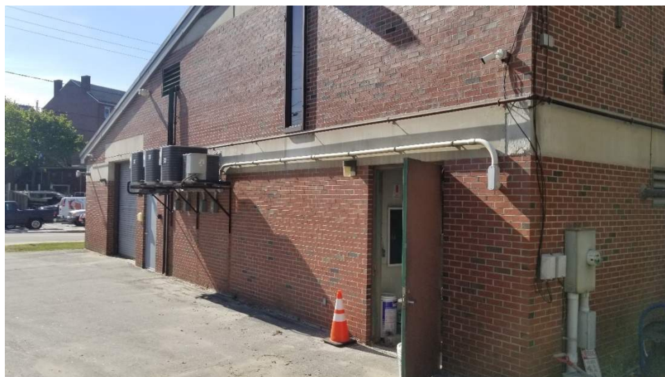
Exposed Gas Pipe at Top of Concrete Band
