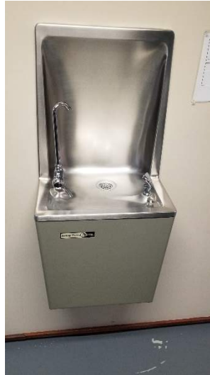
Second Floor Water Cooler
