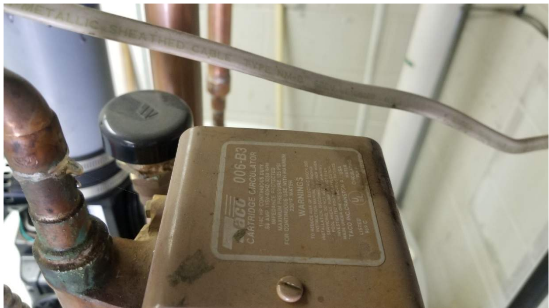
Circulating Pump Nameplate for Domestic Hot Water Return
