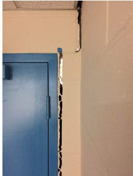
Extensive cracking at stairwell
