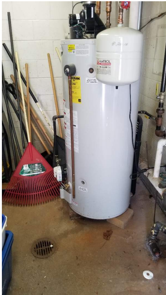
Gas Fired Water Heater
