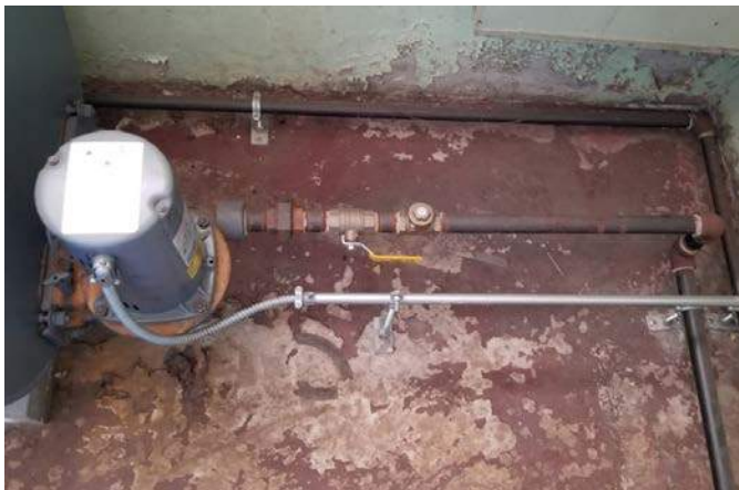
Feedwater pump on back of feedwater tank
