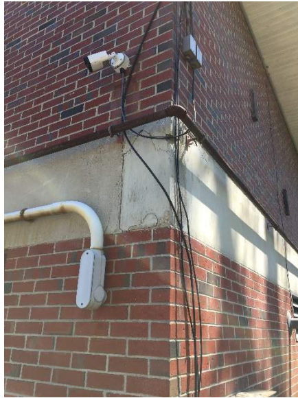
Cracking at precast concrete
