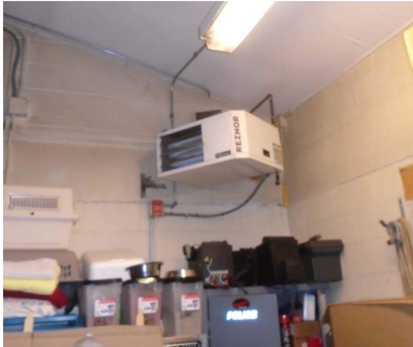
Unit heater in cruiser garage
