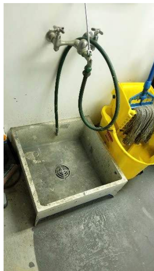
First Floor Mop Basin
