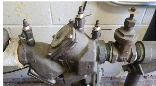
RPZ Backflow Preventer
