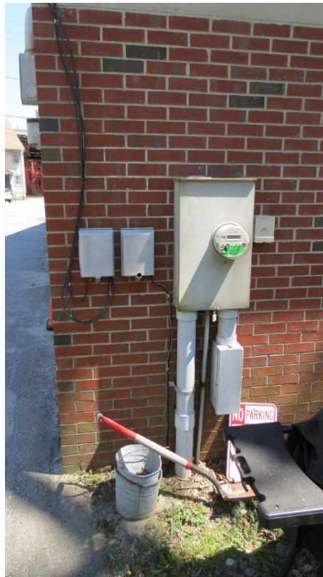
Service entrance meter
