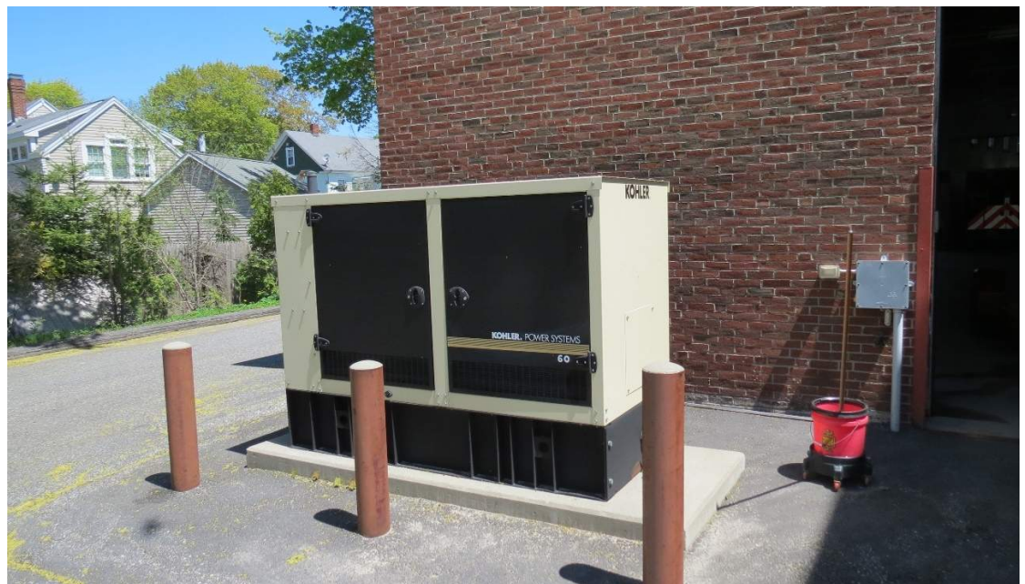
60kw Diesel Generator – Kohler Power Systems
