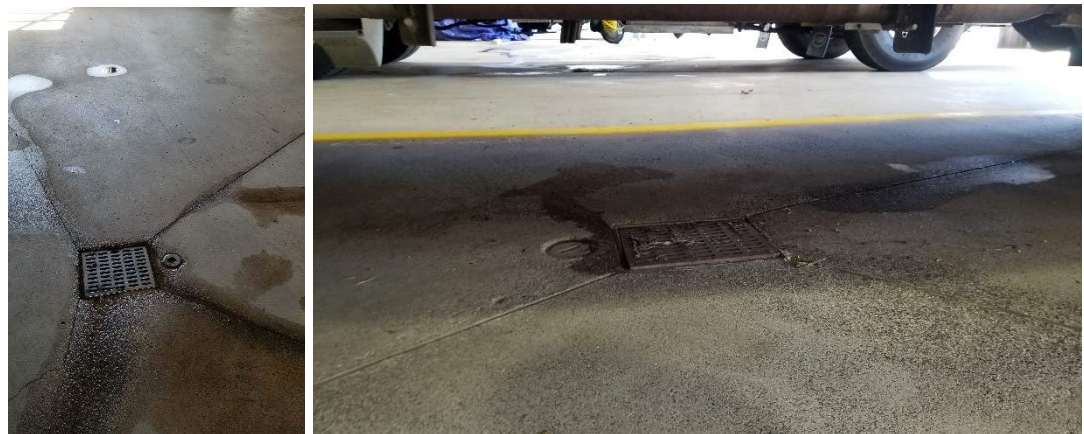
Garage Floor Drains
