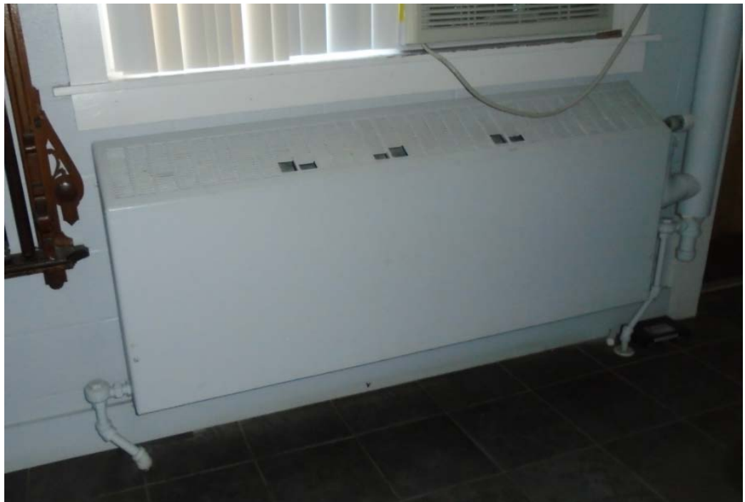
Typical Steam Radiator
