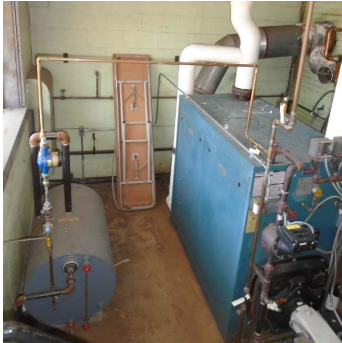
Feedwater tank and controller
