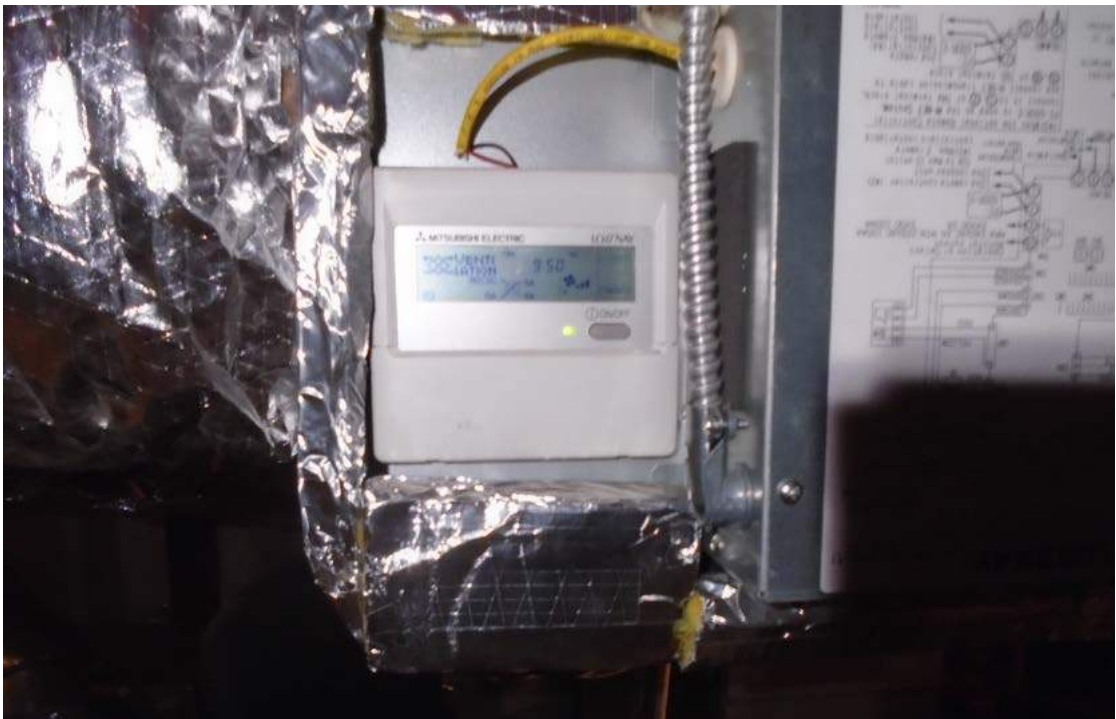
Lossnay main controller installed on unit in attic
