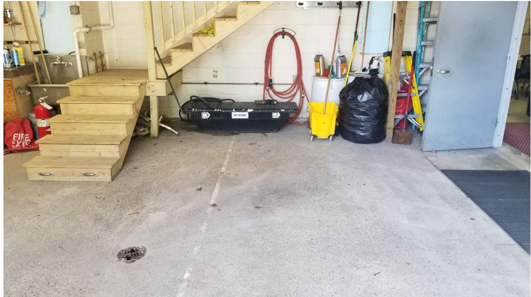
Floor Drain with Service Sink, Condensate Drain from Air Handlers
