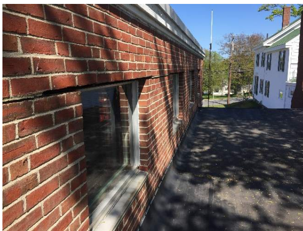
Cracking at lintel locations
