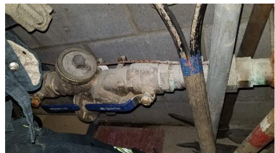
RPZ Backflow Preventer
