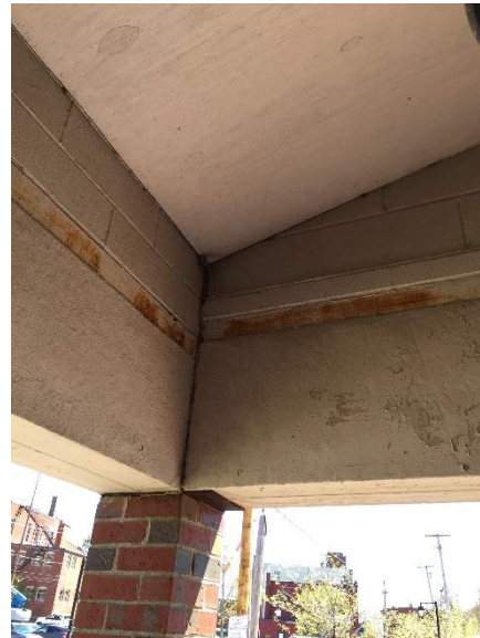
Lintel rusting and spalling of precast concrete at main entry
