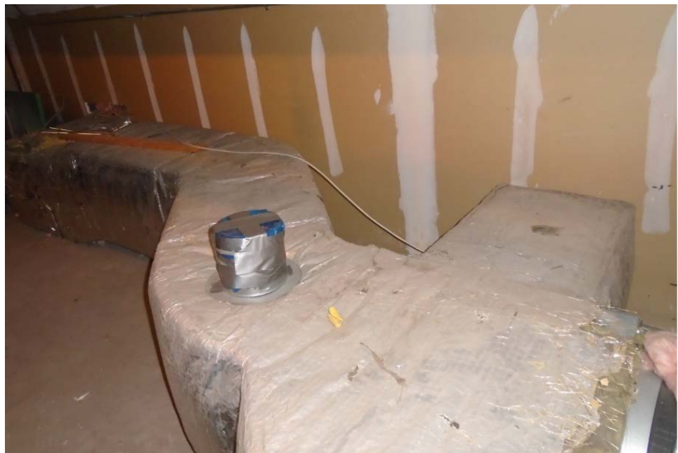
Examples of ductwork in attic
