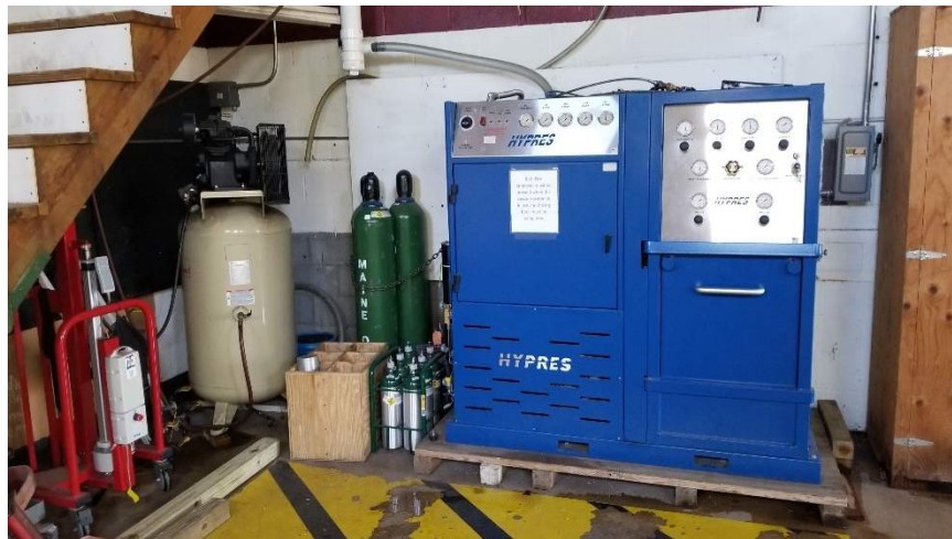
Air Compressor and Breathing Air Compressor with Oxygen Storage (green) Cylinders.
