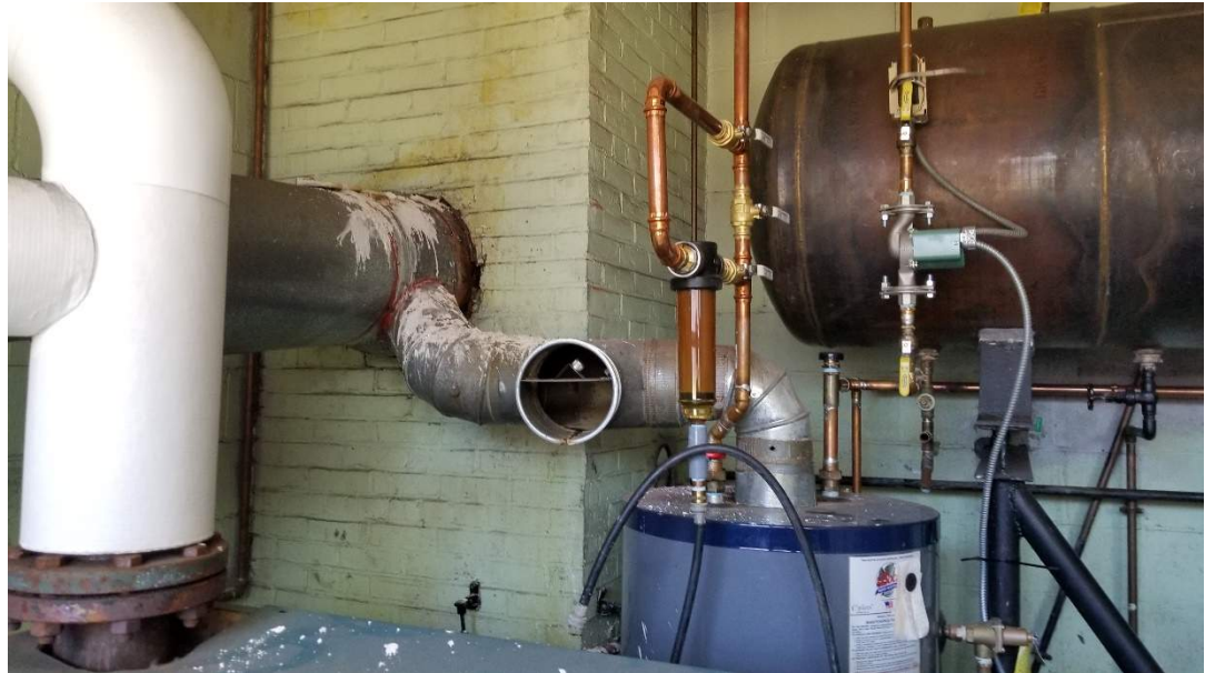
Water Heater Exhaust Flue
