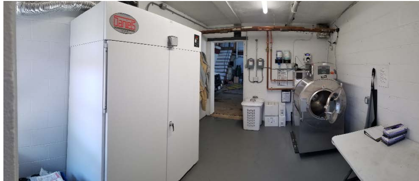
Heavy Duty Gear Washer and Gear Dryer (Note: Un-insulated piping over washer)
