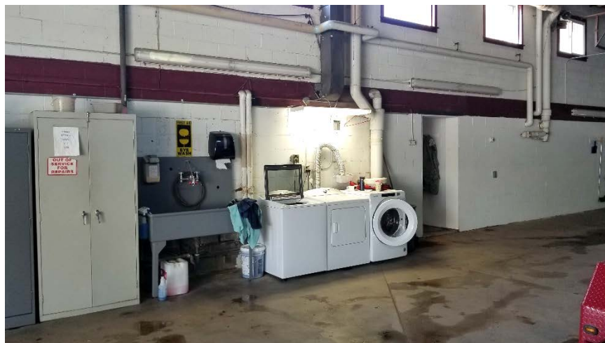
Wash Sink and General Laundry Equipment
