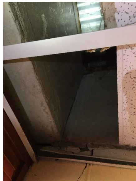
Cracking at exterior wall corner
