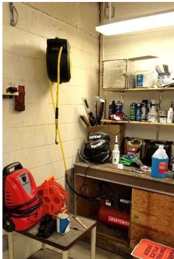
Air Compressor and Hose Reel
