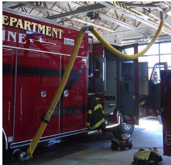
Vehicle exhaust collection ductwork
